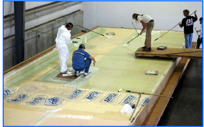
Photo of fabrication of composite main deck (above) by James Betts Enterprises.
